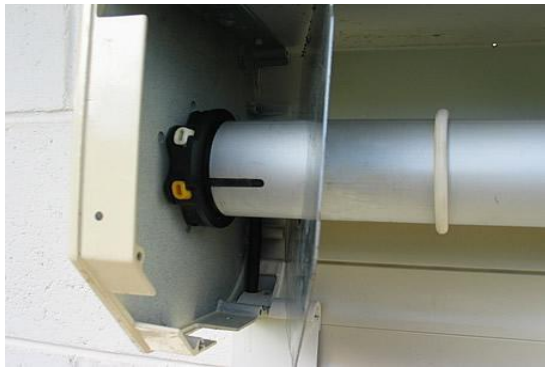
electric motor on left side of roller shutter
